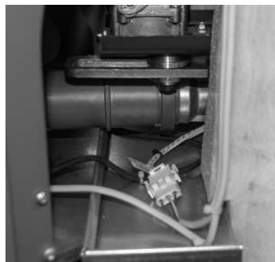
Fig. 59 Elongated sleeve attached to intake pipe at burner.
