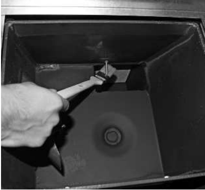
Fig. 37 Clean the thermocontrol sensor
